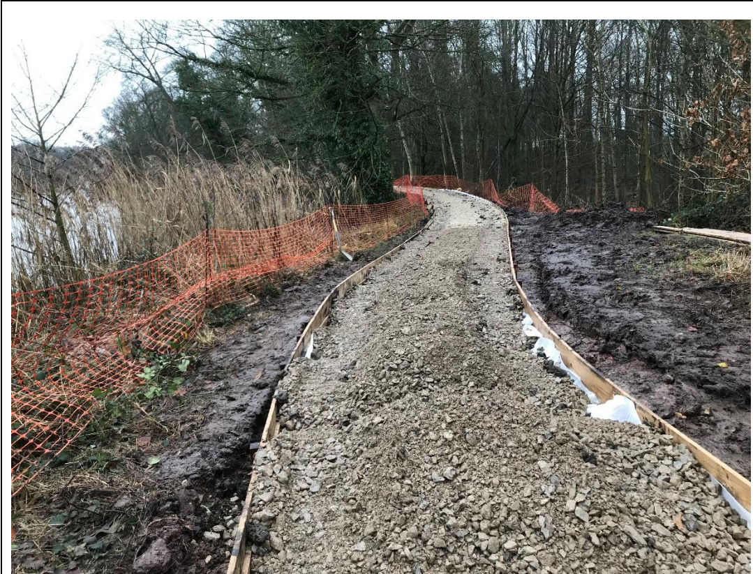
Photograph 3: Raising of dam crest - Tabley Mere, Cheshire (note this is for a relatively small raising of c. 0,2 metres), January 2022 during construction.
