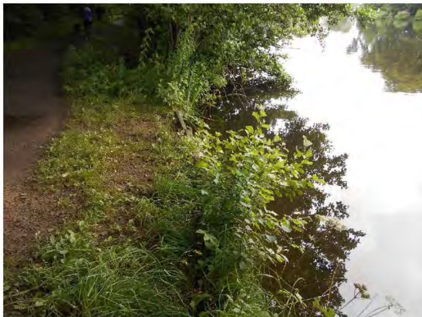
Photograph A2: Section of upstream edge of the crest with timber revetment providing support
