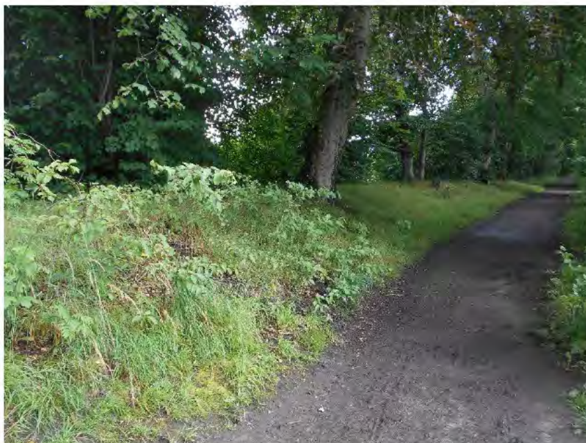
Photograph A4: Crest of dam towards south end with raised area at the downstream side
