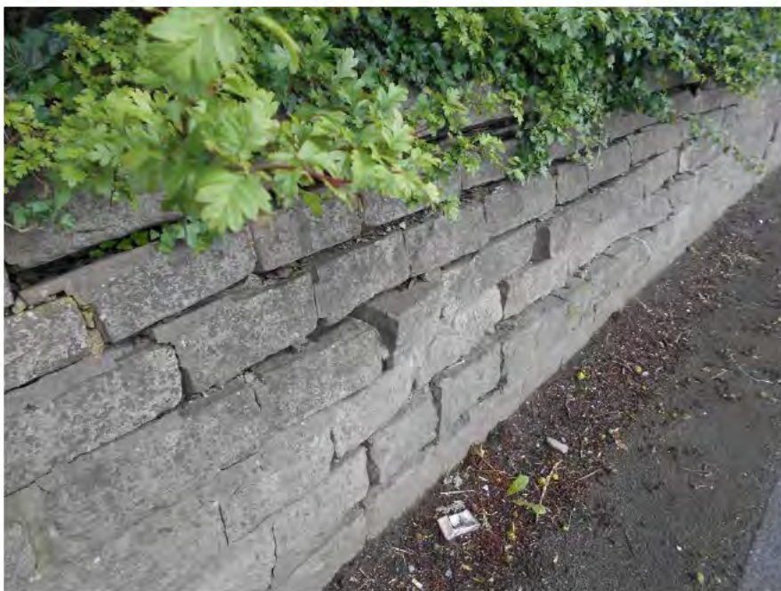
Photograph A8: Bulging and displaced stonework within the wall
