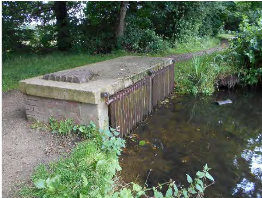
Photograph A11: Inlet structure with screen at the upstream end of the overflow pipe
