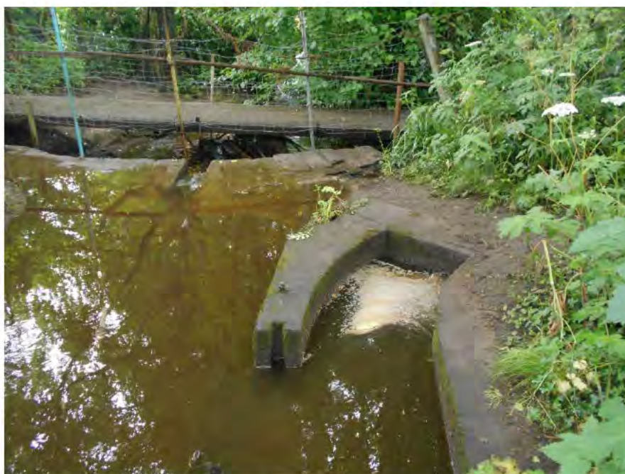
Photograph A14: Weir and bifurcation structure on the Poynton Brook at upstream side of Parklands Way
