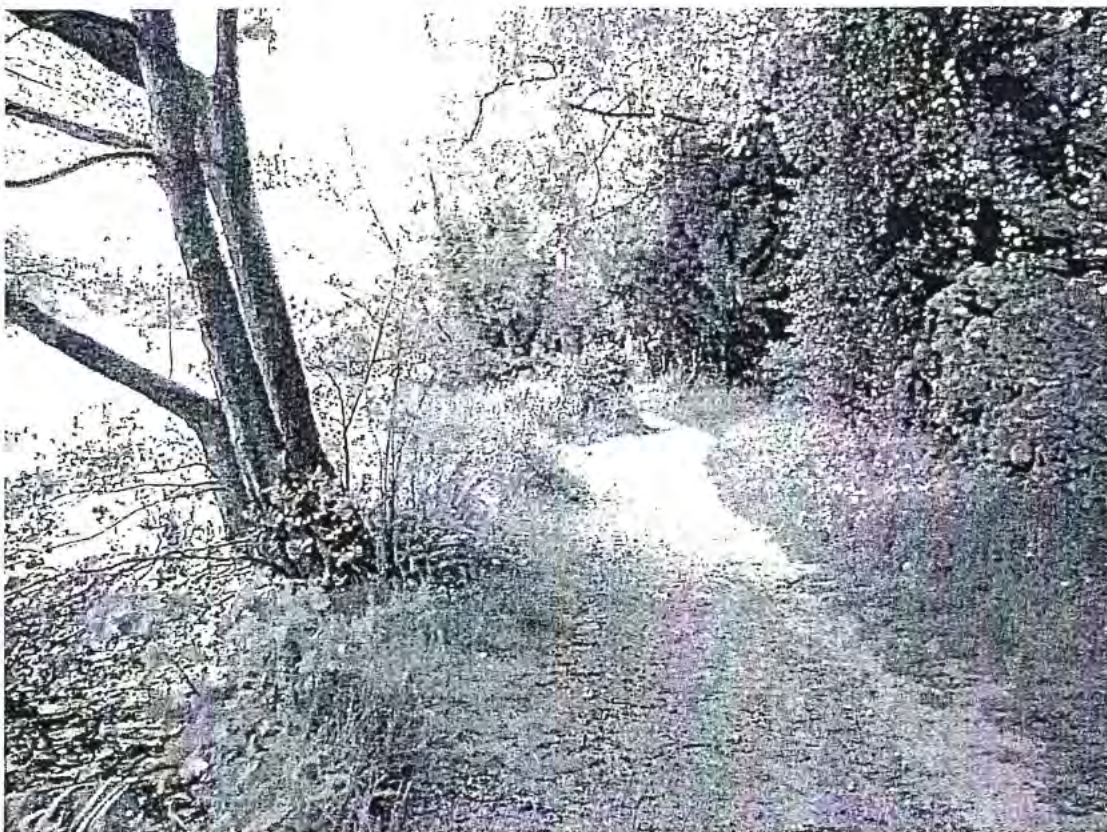
Photograph 5 – Leaning tree on dam crest
